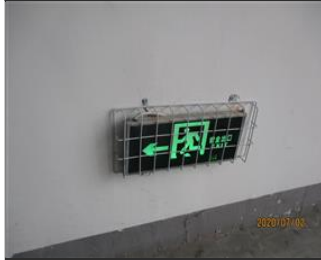
Photo of fire safety equipment Evacuation sign.JPG
