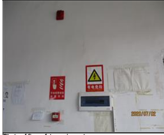
Photo of fire safety equipment Fire alarm.JPG
