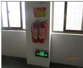
Photo of fire safety equipment Fire extinguishers.JPG
